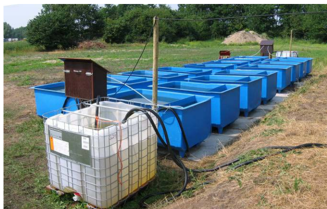
STP Horstermeer, The Netherlands Rather high loaded activated sludge process
