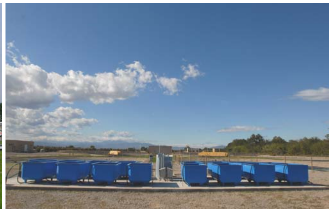
STP Empuriabrava, Costa Brava, Spain Very low loaded activated sludge (oxidation ditch)
